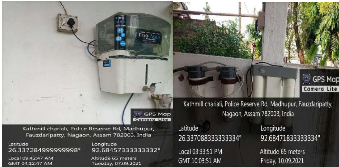
Figure 44: Drinking Water Facility
