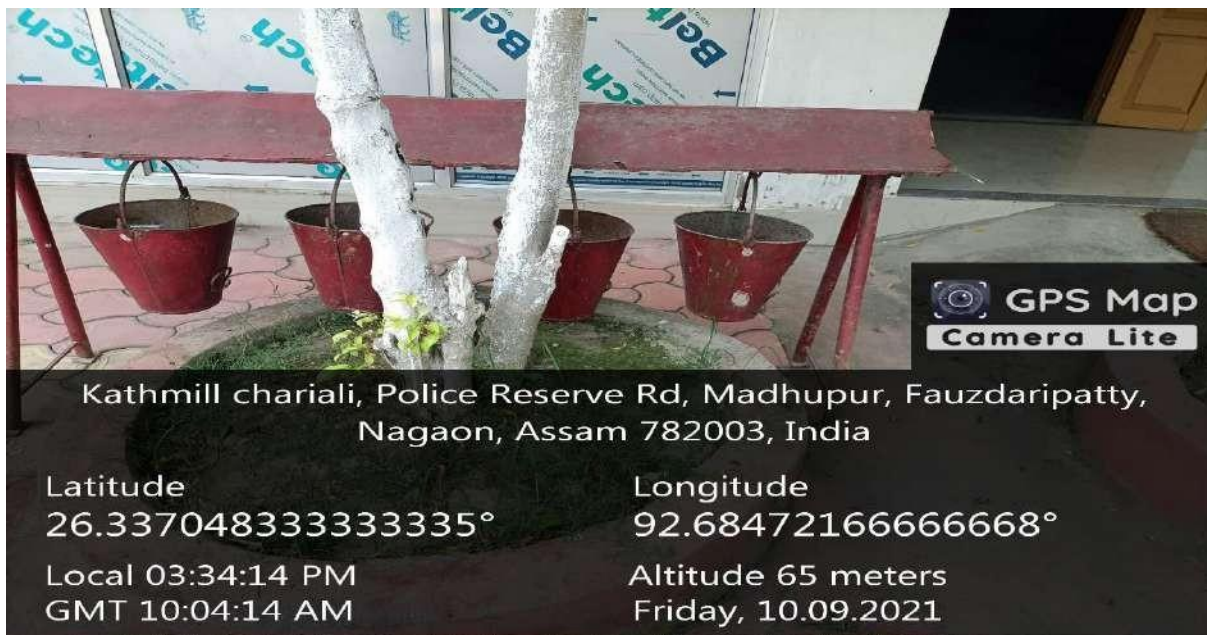
Figure 49: Fire Extinguisher Bucket
